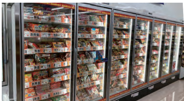
Interior of store with energy-conserving refrigerators/freezers
