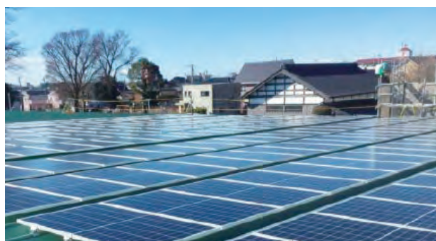
Store outfitted with solar panels
