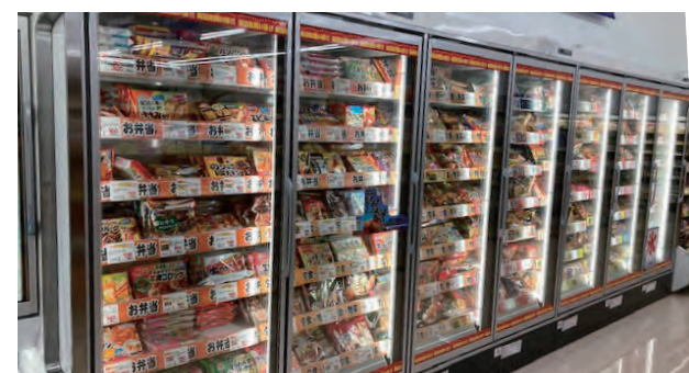
Interior of store with energy-conserving refrigerators/freezers
