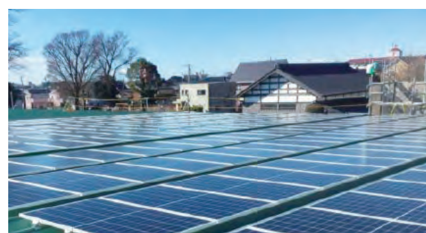
Store outfitted with solar panels
